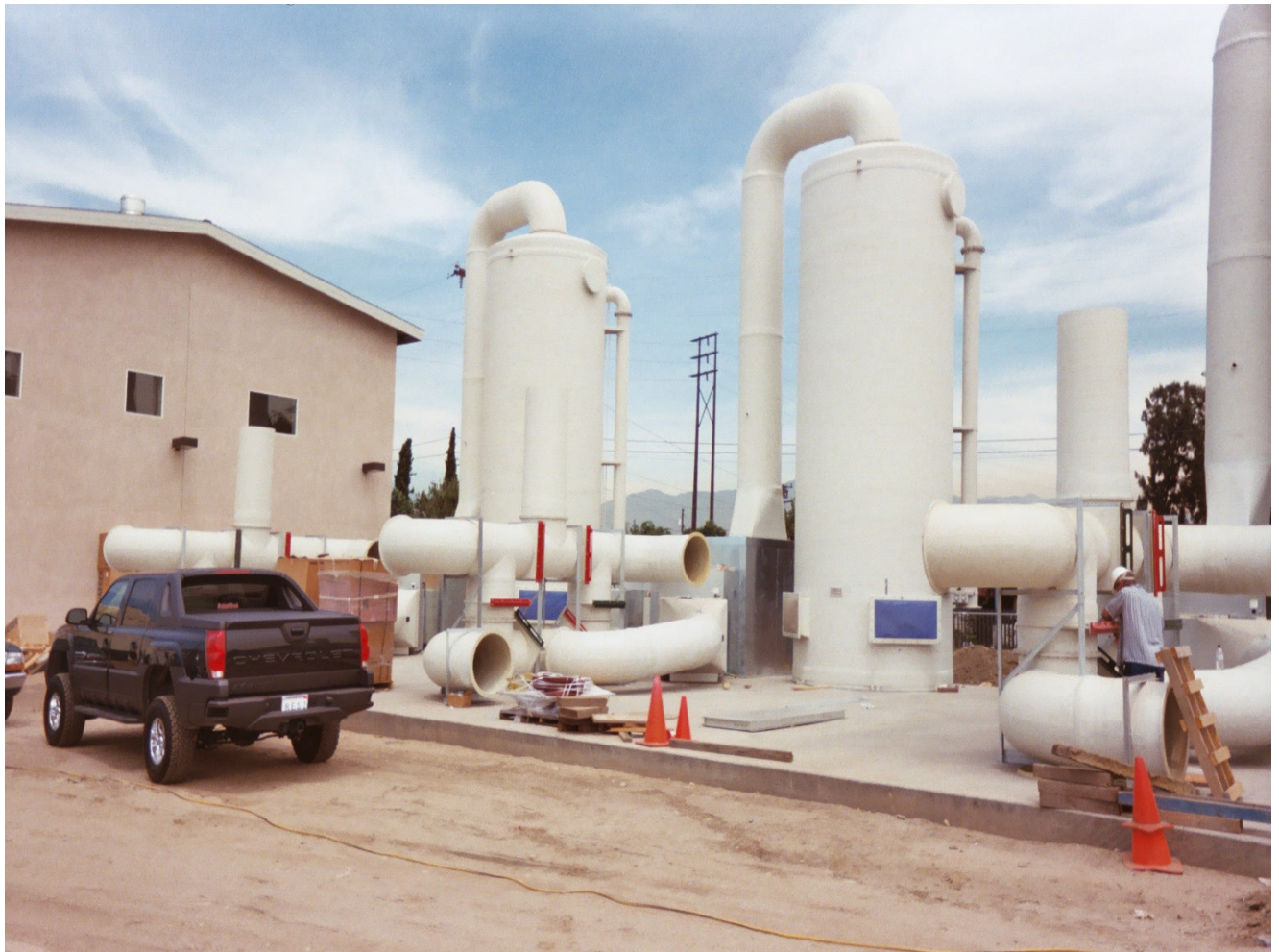
B6-San Gabriel Valley Water District Project Four (4) 10-foot diameter ACS Air Stripper Towers with FRP Ductwork
